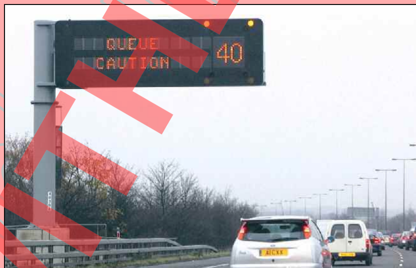
Figure 2. Two Line Motorway Signal Mark 3 (MS3) - the MS4 is an alternative to this MS3
