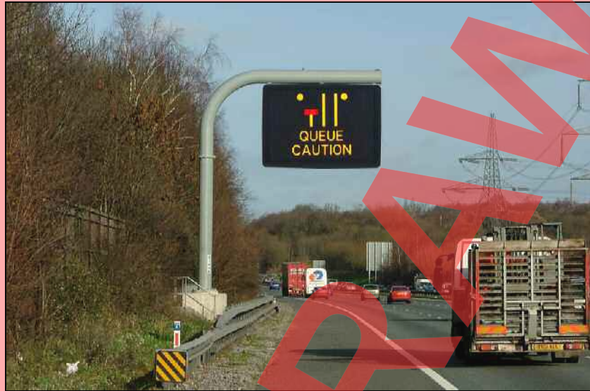
Figure 1. Motorway Signal Mark 4 (MS4)
