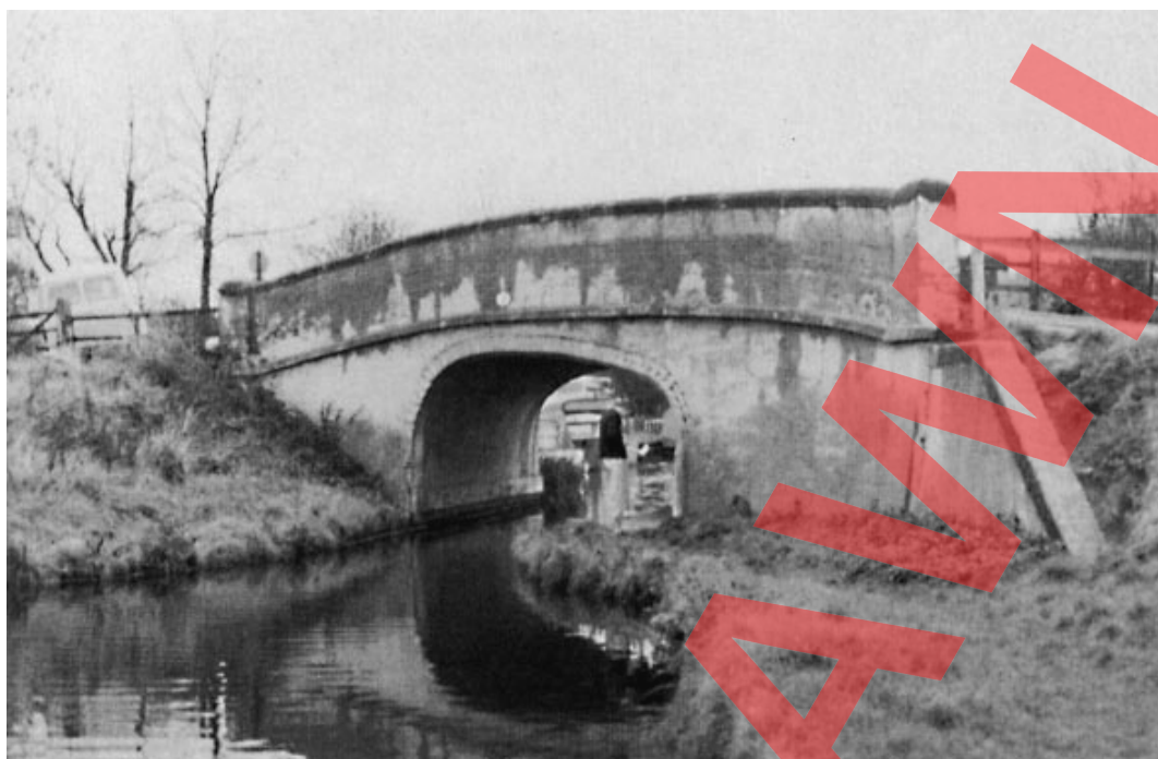
Plate 6 This shows an arch which has become grossly deformed and flattened in shape. The MEXE method would not be suitable for assessing its carrying capacity and instead it should be assessed from first principles.
