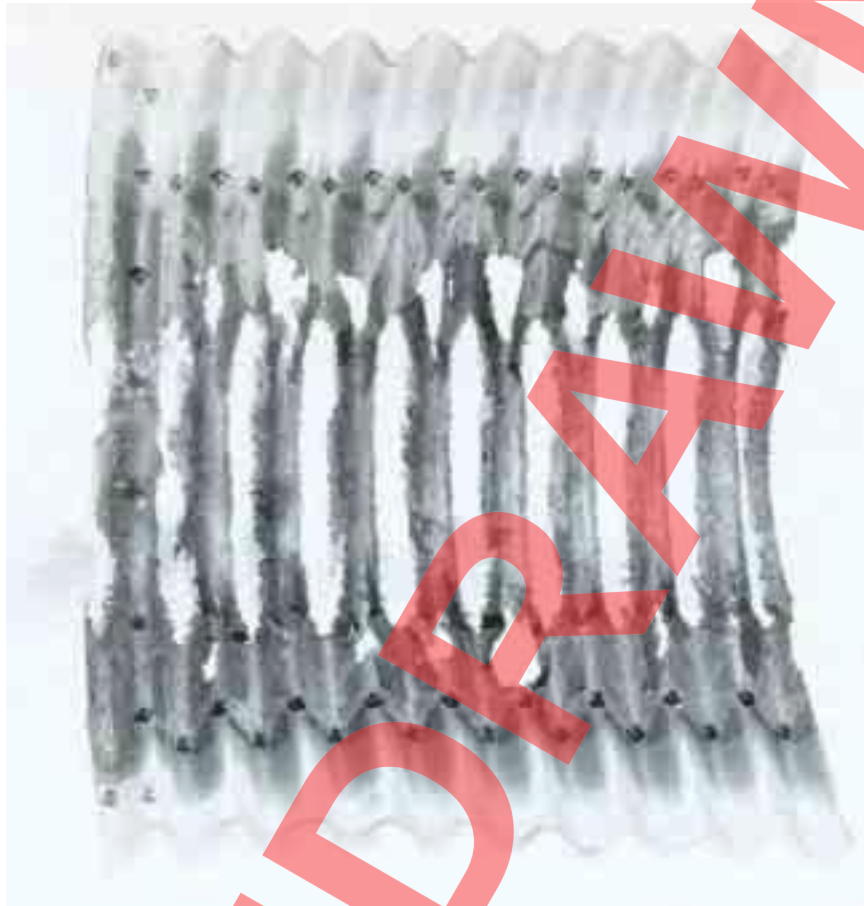
Figure B.1 Example of extreme corrosion in the invert of a structure subject to scour (this 30 year old structure was not provided with a paving or bitumen coating)
