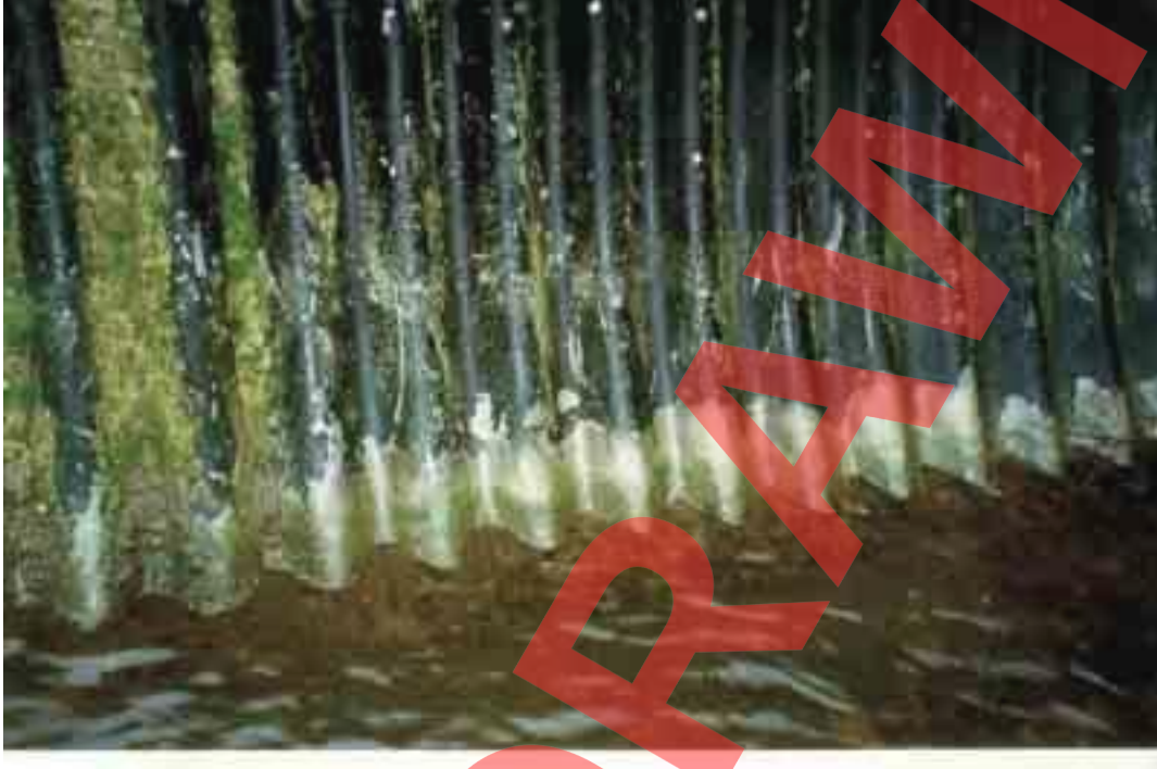
Figure B.2 Deterioration of bitumen coating along the wet/dry line in low flow condition
