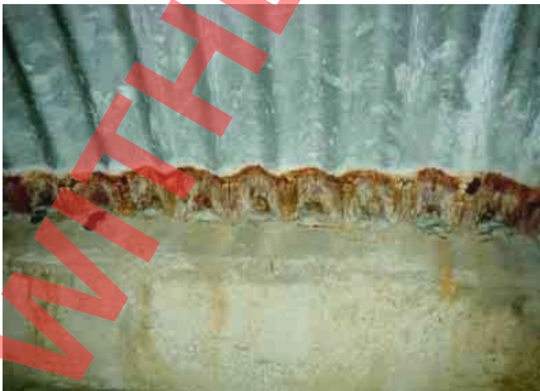
Figure B.9 Deterioration at the arch seating of a plain galvanised arch structure due to seepage and ponding of water containing de-icing salts
