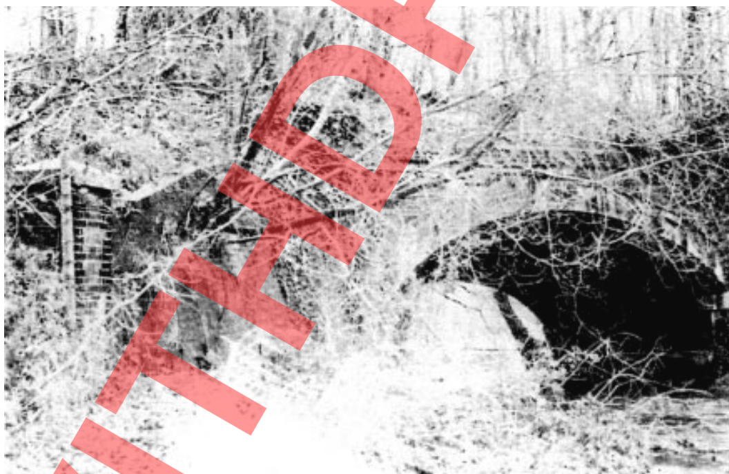
Plate 12 This shows vegetation growing from the faces of the bridge and wing walls; this vegetation should be cut back before it has a chance to damage the brickwork.
