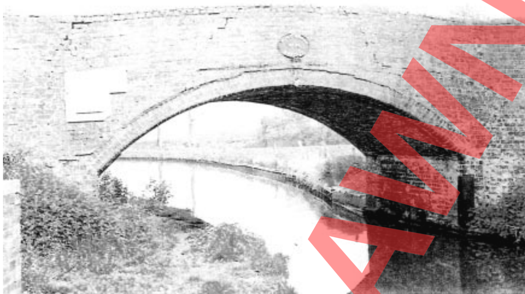
Plate 11 This shows cracking of the spandrel/parapet walls which suggest a flexible arch barrel.
