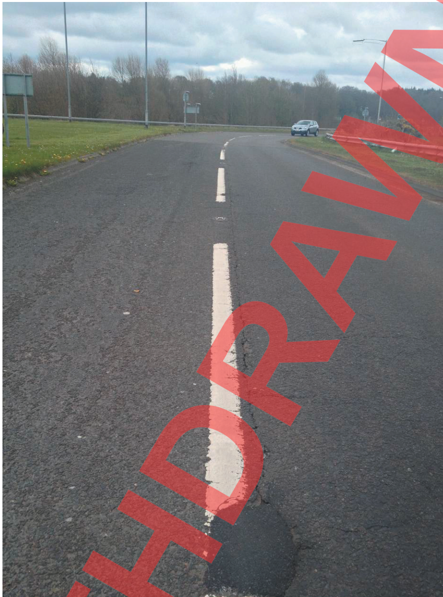
Figure E5: Condition Score 40 – long view
