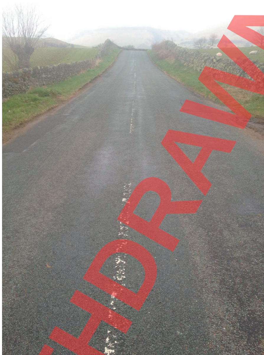
Figure E14: Condition Score 0 – long view
