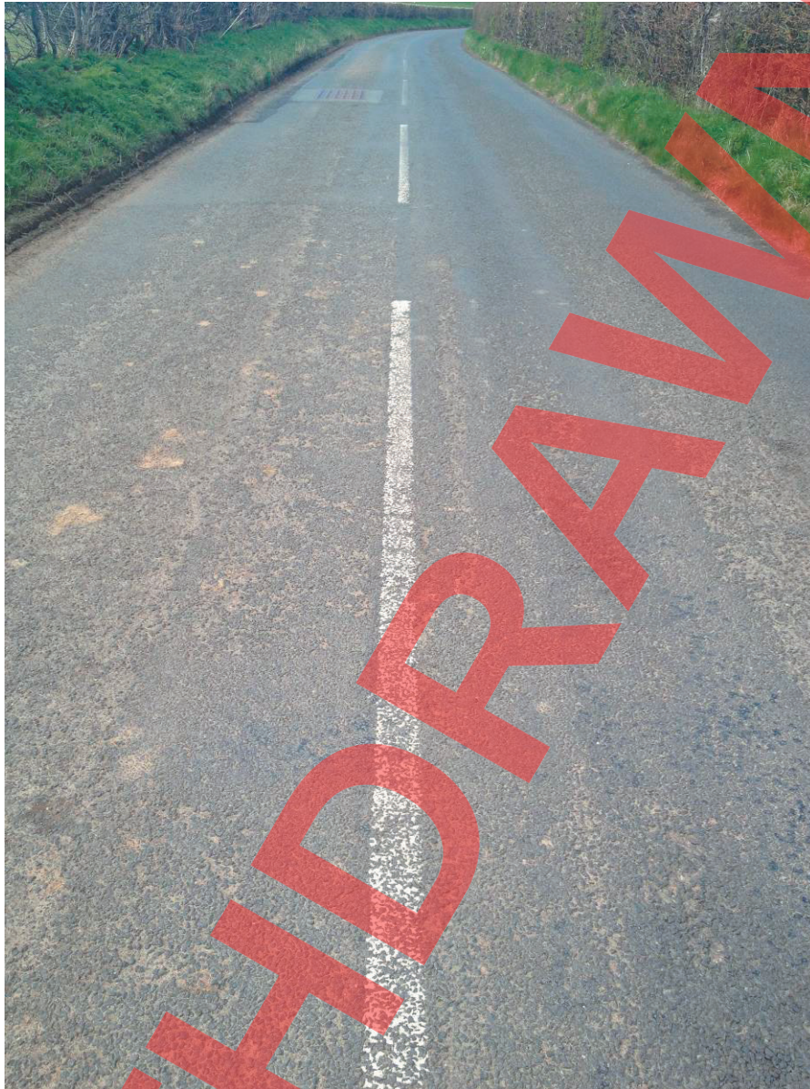
Figure E12: Condition Score 10 – long view
