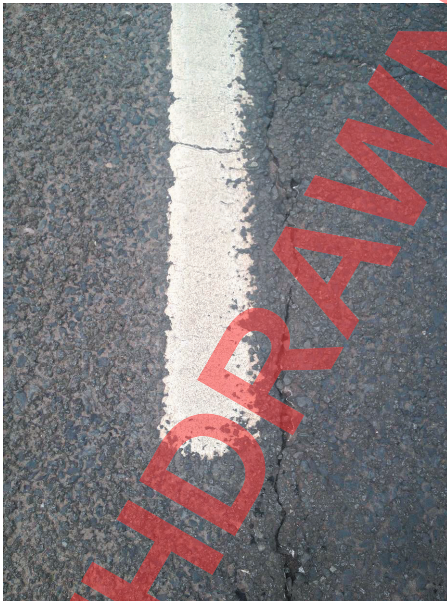
Figure E4: Condition Score 40 – close-up
