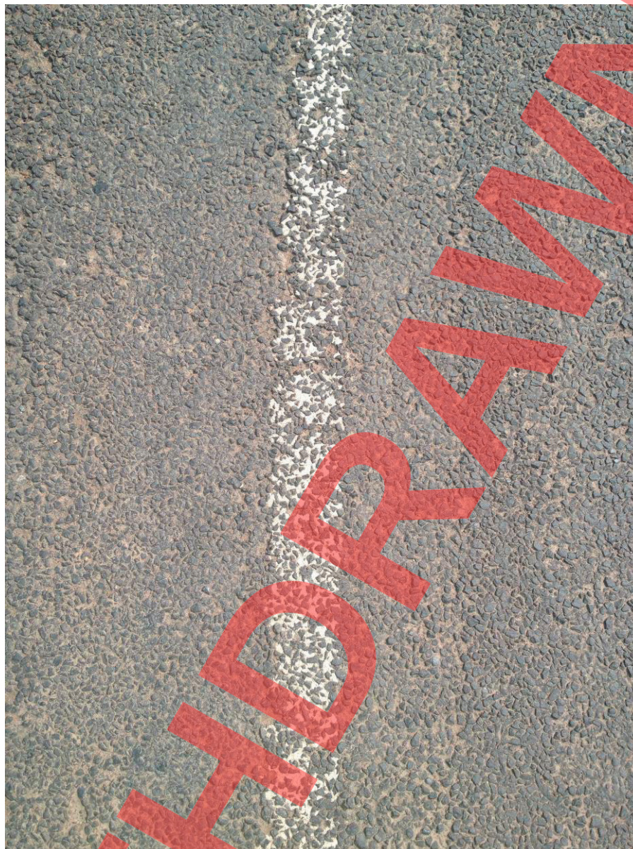
Figure E11: Condition Score 10 – close-up
