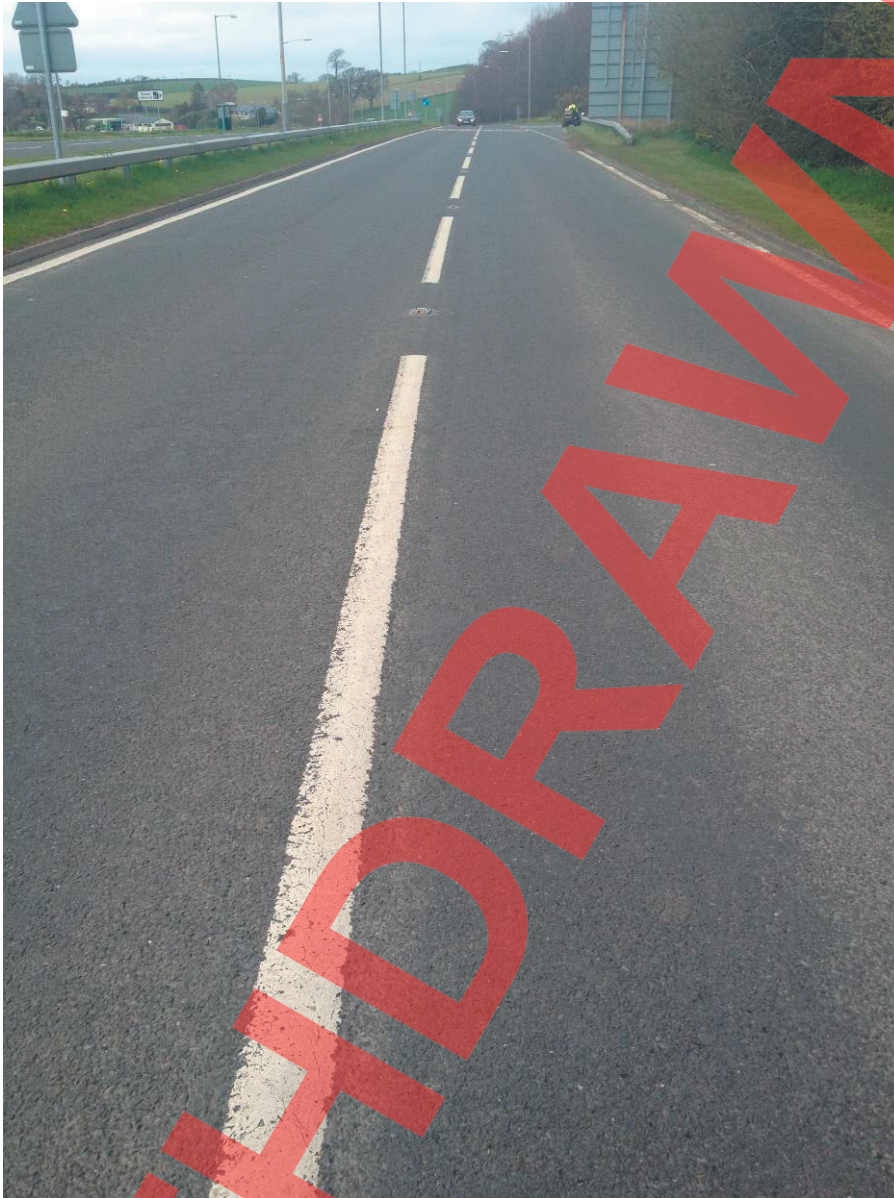
Figure E7: Condition Score 30 – long view
