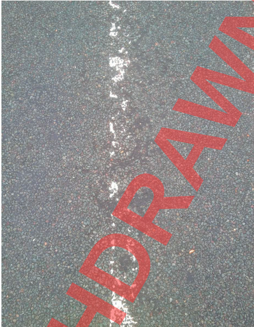
Figure E13: Condition Score 0 – close-up
