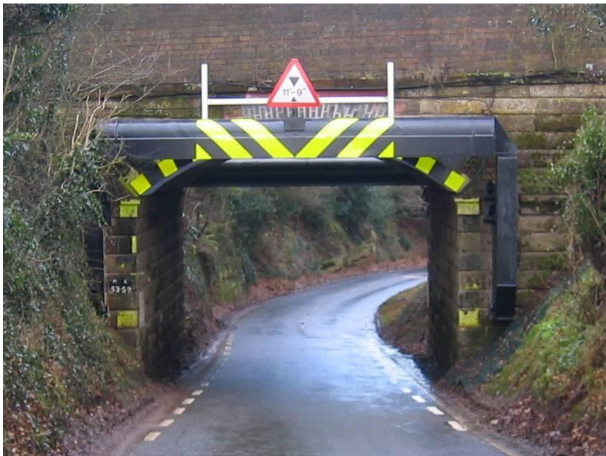
Figure A.7 Collision protection beam to arch at height of chord markers
