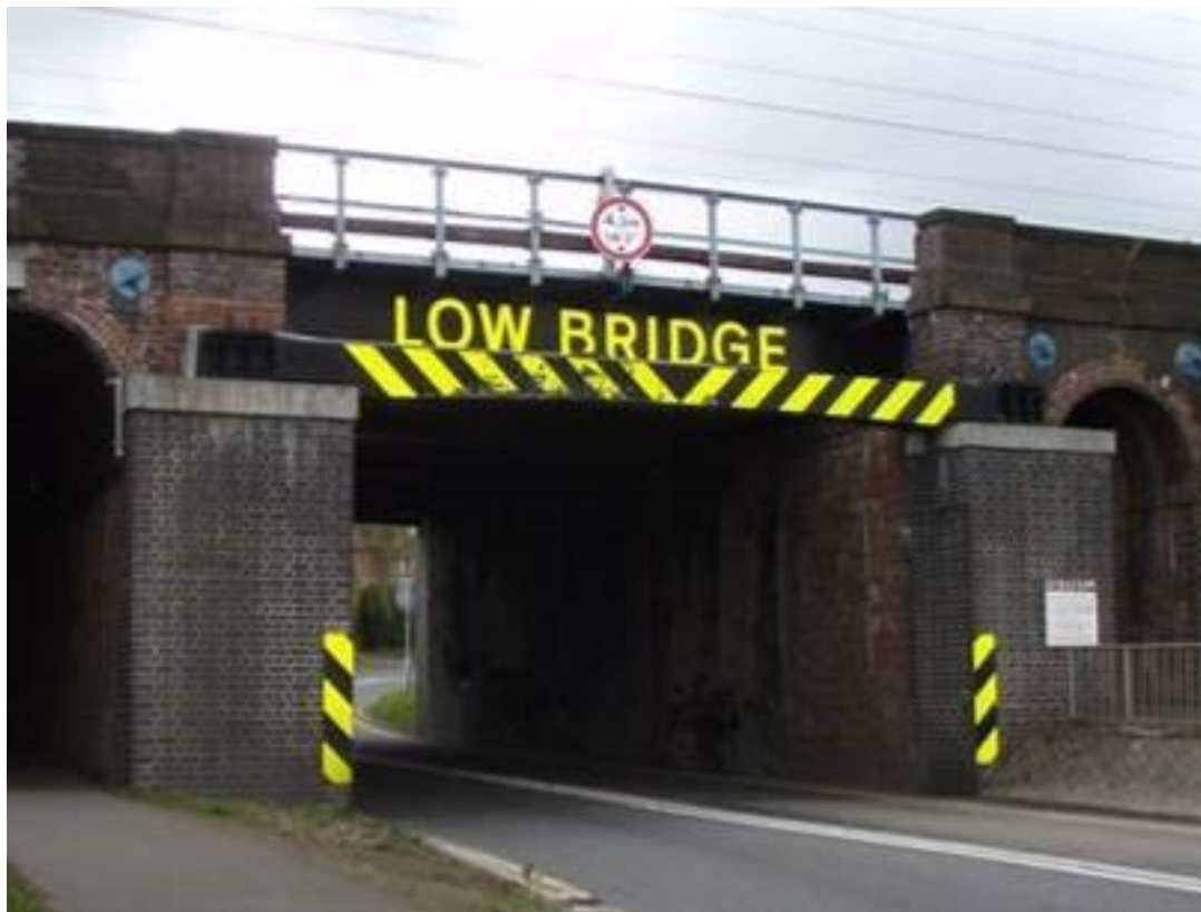
Figure A.6 Collision protection beam to flat soffit bridge supported from abutment extensions. Note the camber to the beam
