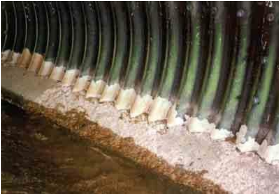
Figure B4 shows, the details of raising the sides of paving within a pipe arch structure that was constructed with a flat reinforced concrete paving.
