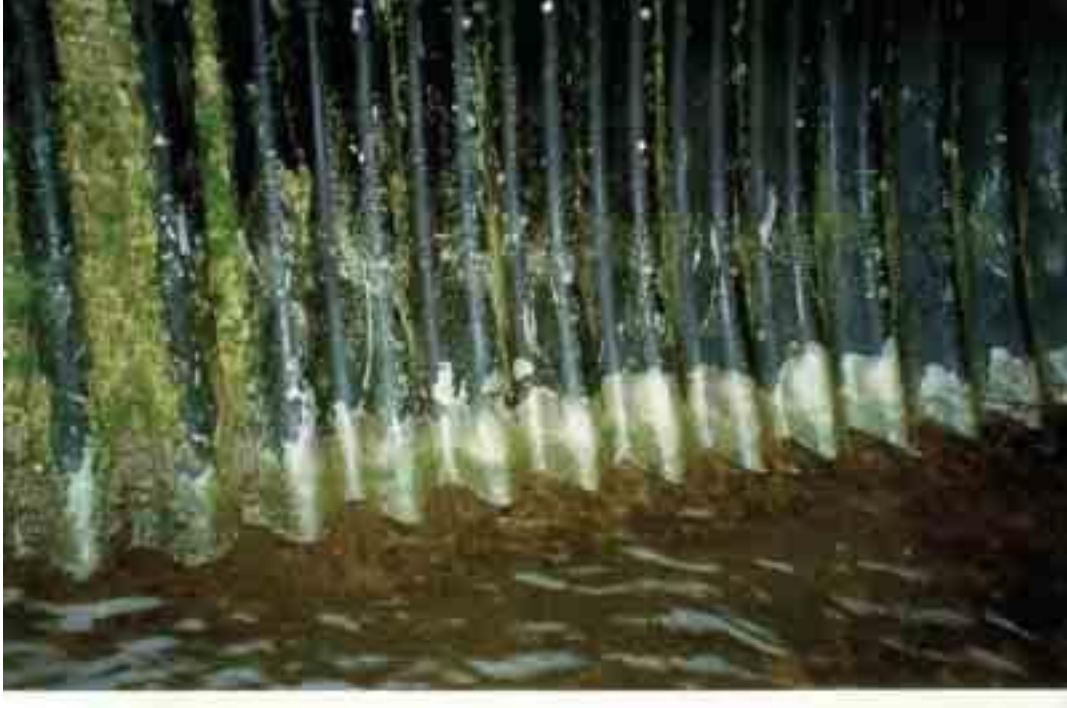
Figure B.3 Damaged bitumen coating caused by overtopping of paving during turbulent flow
