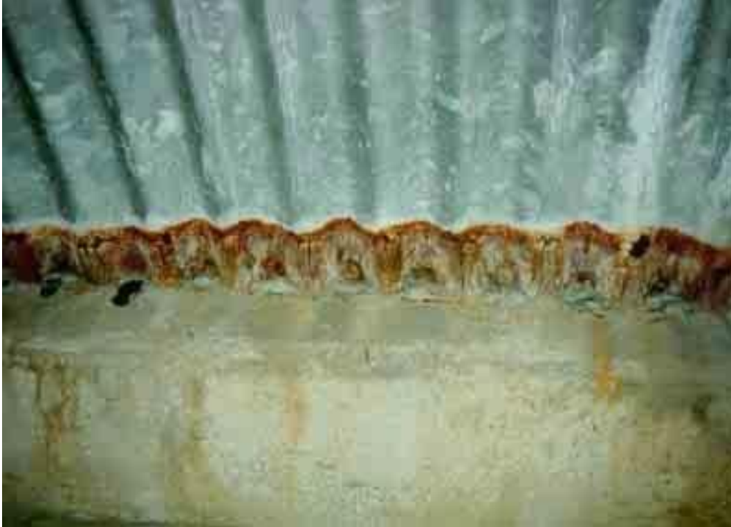
Figure B.9 Deterioration at the arch seating of a plain galvanised arch structure due to seepage and ponding of water containing de-icing salts
