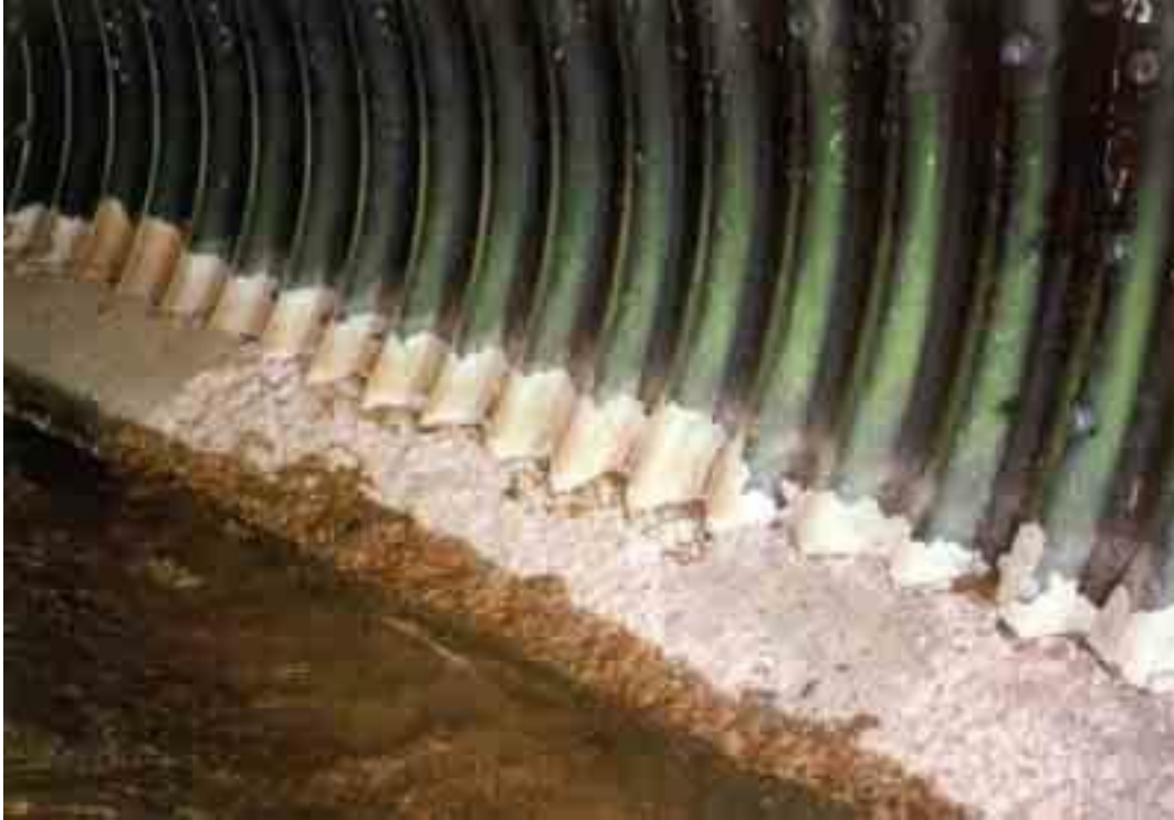
Figure B.11 Damaged bitumen coating caused by overtopping of paving during turbulent flow
